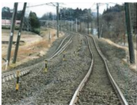
Fig.2 Subsidence of embankment
