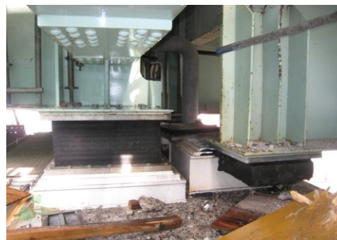
Figure 5 Damage to a bridge support
