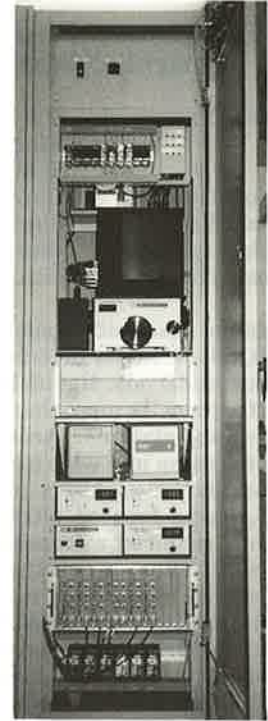
Photograph 1. View of diagnostic cabinet
